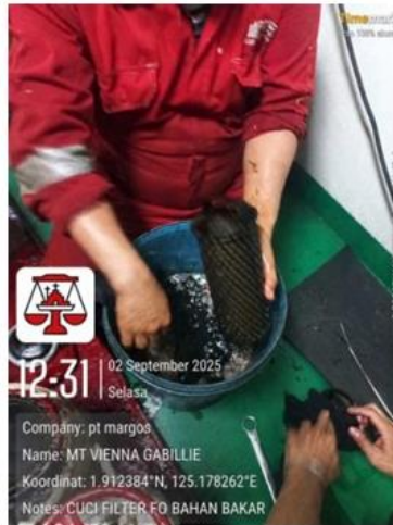
Gambar 4. Cuci Filter Fuel Oil.
